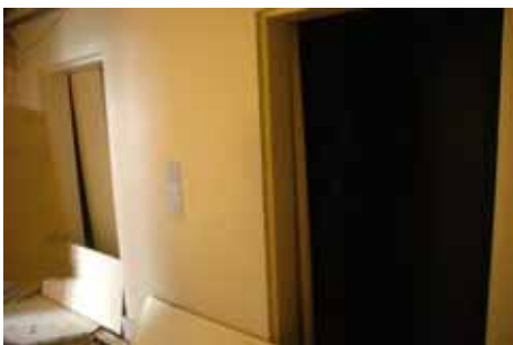
Lift doors blown out
