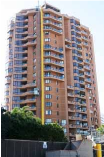
Repair work will take some months to complete
