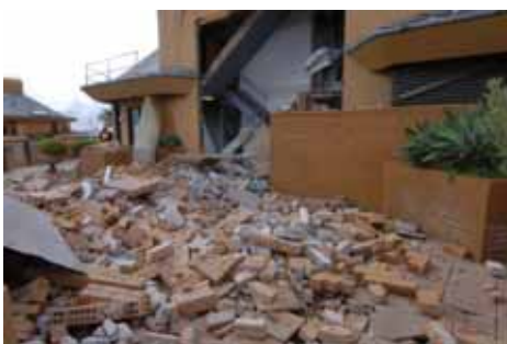
Masonry walls blown out
