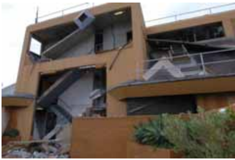
Damage to plant areas
